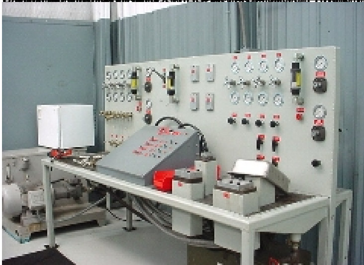
Control panel for the repair of heavy machinery and large components.
